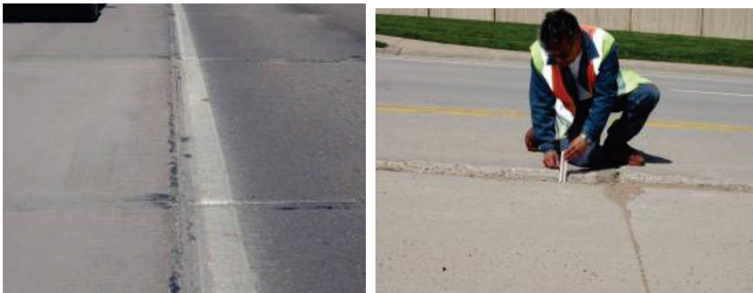
Figure 7. Longitudinal joint faulting on I-25 (left) and Wildcat Reserve Parkway (right) in the Denver area.
