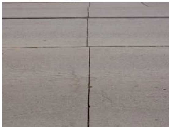
Figure 8. Slab slippage due to inadequate design or placement of tie bars between adjacent lanes on Broadway Avenue in Douglas County, Colorado.
